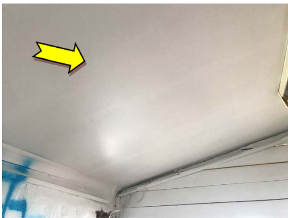
Photo 5. Interior, throughout, ceiling – suspected lead-containing white upper paint system.
