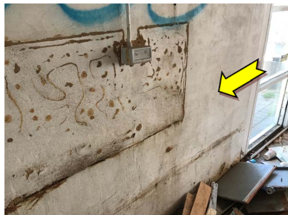
Photo 6. Interior, throughout, walls – suspected lead-containing white upper paint system.
