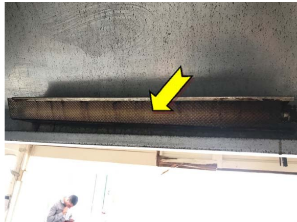
Photo 4. Interior, throughout, single tube light fittings – suspected PCB containing capacitors.
