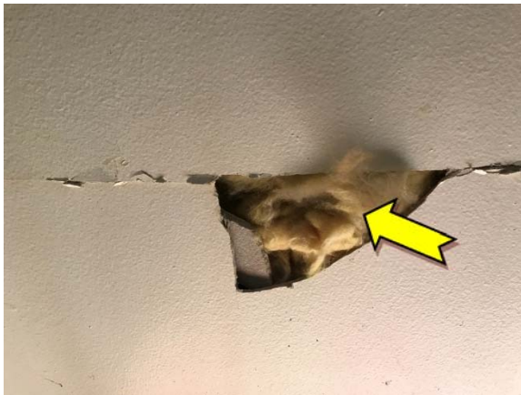
Photo 3. Interior, throughout ceiling space, sarking insulation – suspected SMF.
